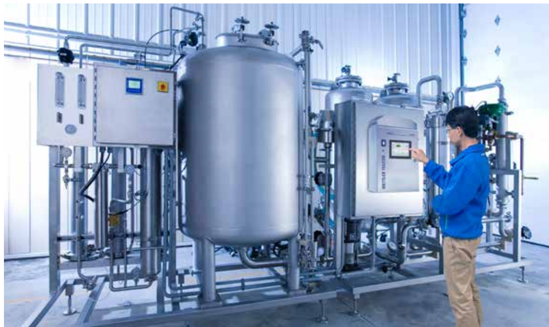
Field service engineer is commissioning the 7000RMS installed on the water system skid.
